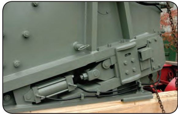
Hydraulic cylinders do the heavy work. Lightweight shims are inserted from the side where access is best.
